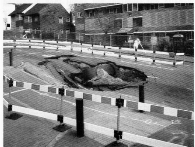
The 2002 big hole in the A2 carriageway, with a broken water main in its middle. Photo John King
